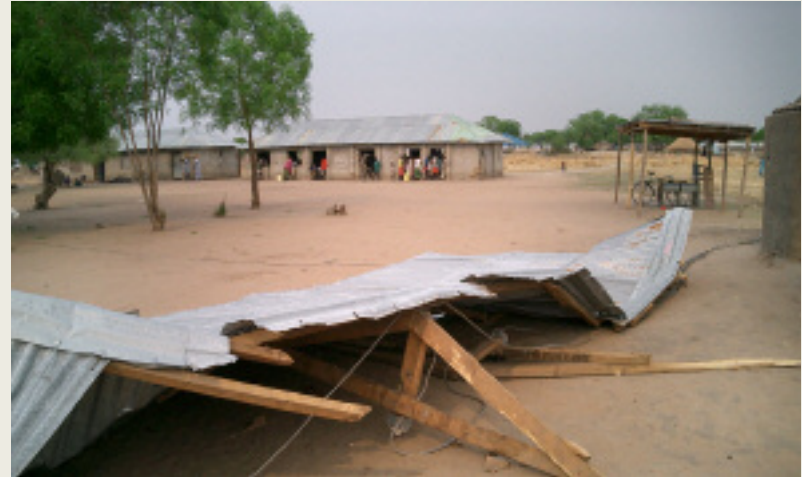
Current condition of Mark Nikkel school in need of serious repair.
